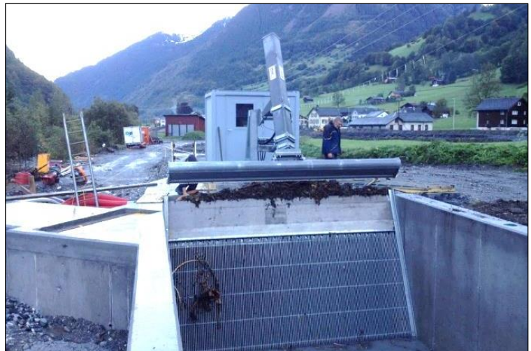
Grill at the end of the sand trap
