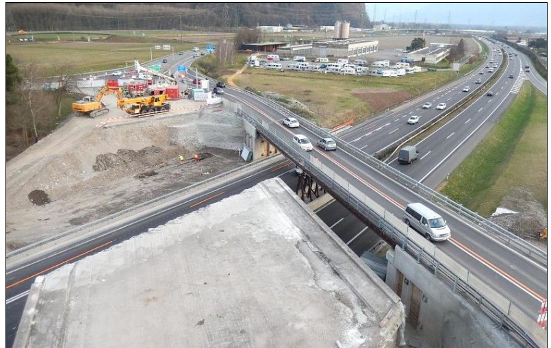
Demolition of existing bridge in two phases, diversion of traffic via cantonal road over provisional bridge
