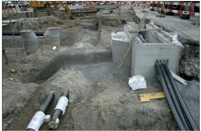
Electricity shaft Murtenstrasse
