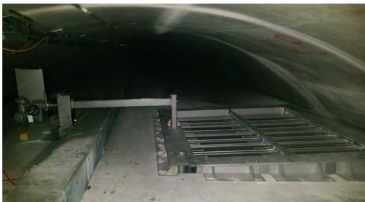
Figure 4: New exhaust air valve
